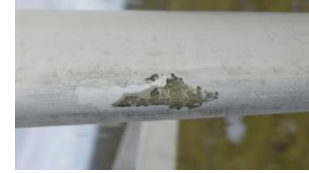
Topcoat damage due to air trapped during the manufacturing process
